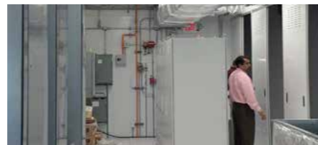
HVAC air ducts
