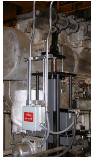
Figure 4. Electric Actuator direct on valve rack
