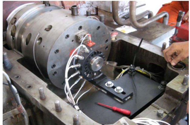
Figure 2. Speed Gear and Speed Sensor Installation
