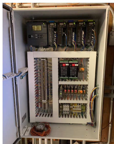
Upgraded kiln cabinet with SLATE combustion controls.
