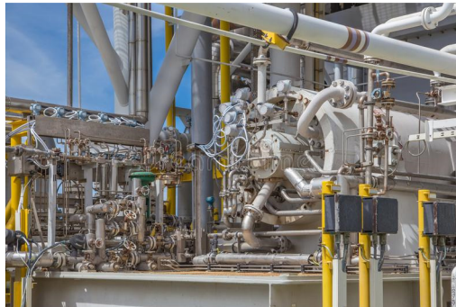
Figure 1: Site operators that are able to shut down one gas turbine can save a significant amount of gas through lower “idling” consumption.
