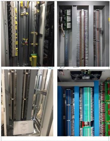
MARSHALLING CABINET - CURRENT
