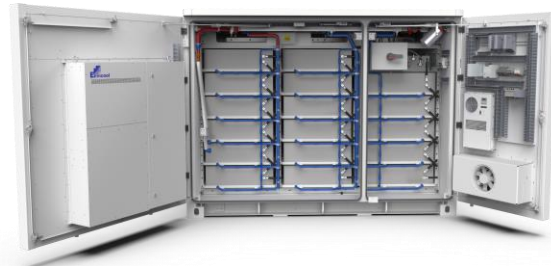
Honeywell offers a variety of battery block and power conversion system (PCS) options
